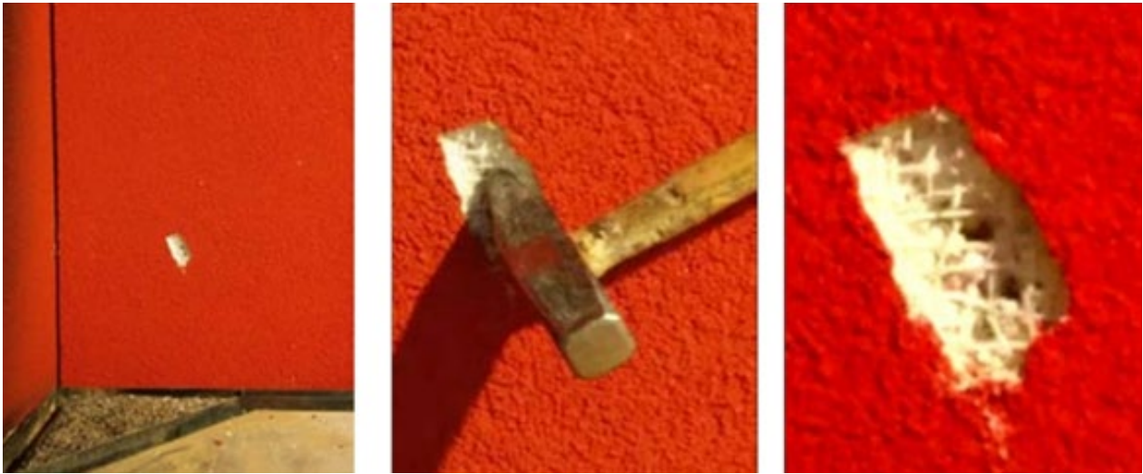
FIG. 3. DAMAGE MANUALLY DONE BY HAMMER ON SAMPLE B2
