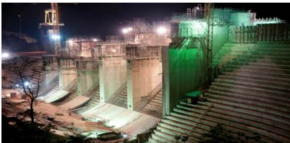
CMC – Sud Africa Ingula Pumped Storage Scheme
