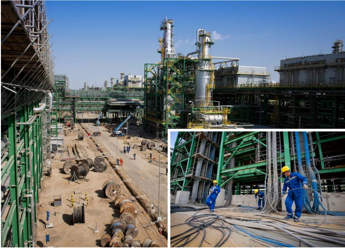
Bonatti - Kashagan Kazakhstan Electrical Instrumentation Works
